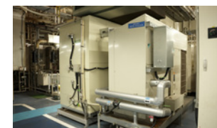
JIZAI HEAT installed at the Rinkai Factory
