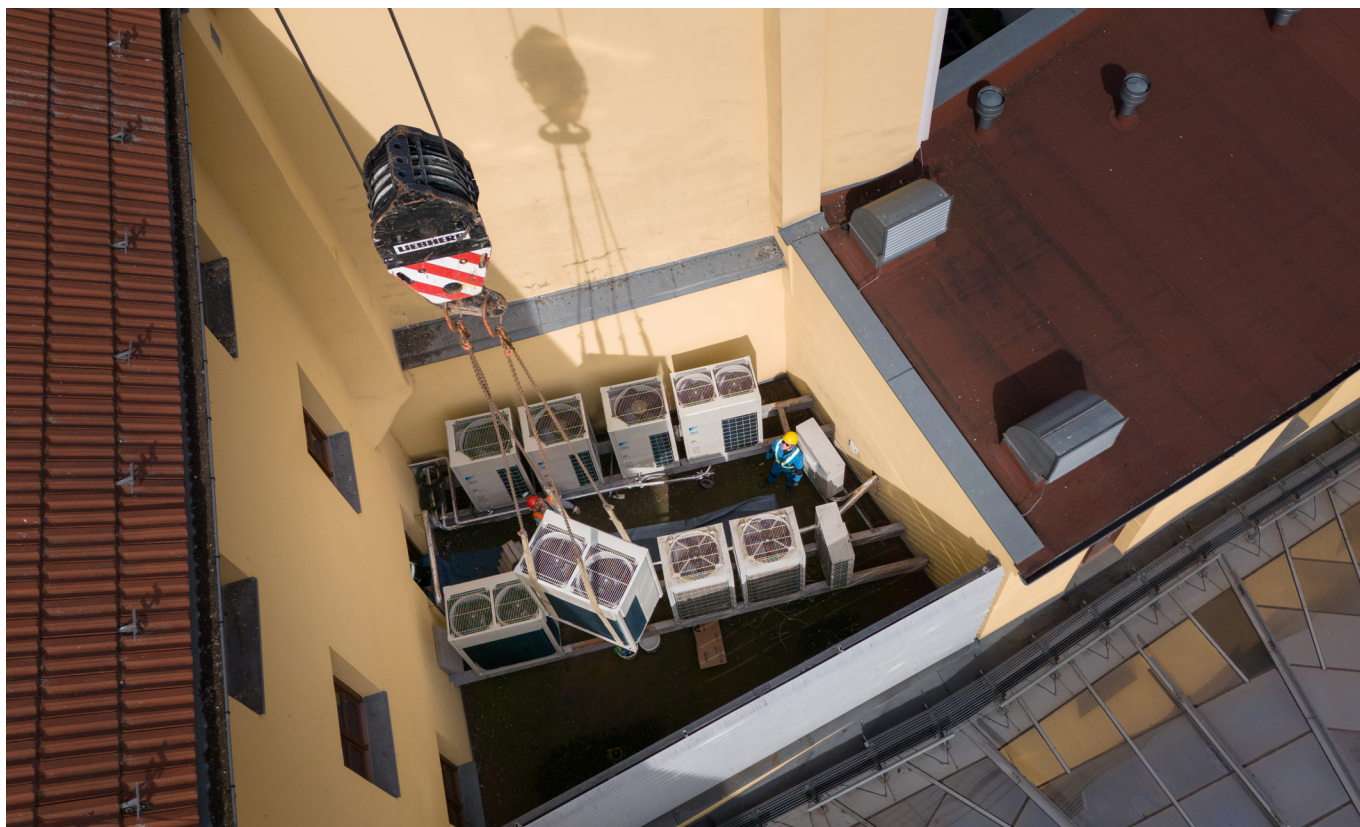
The original VRV III outdoor units served four floors of the building reliably for 15 years.
