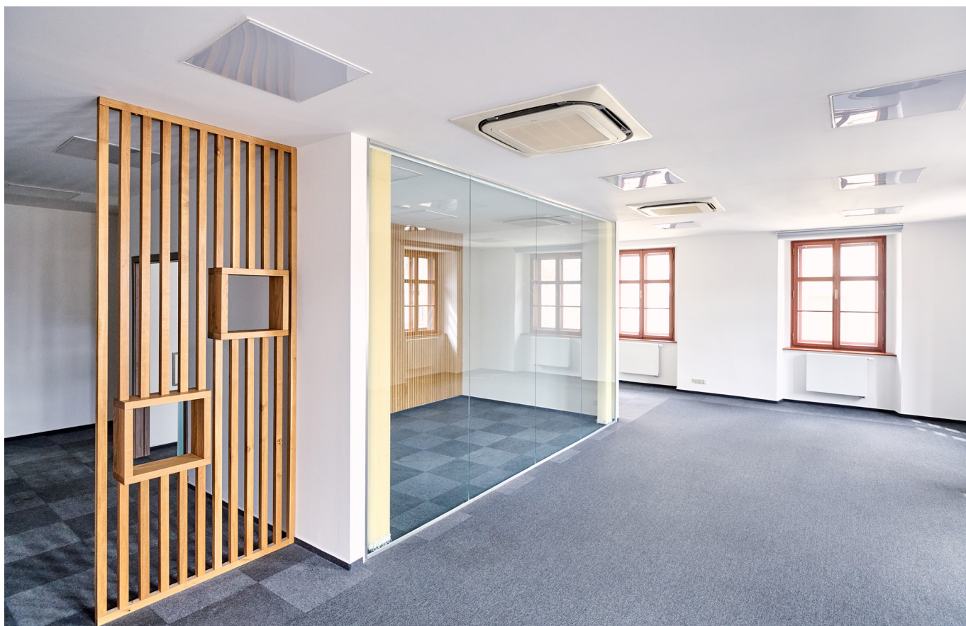
Inside Salm Palace, the original indoor cassette units and interior spaces remained untouched.
