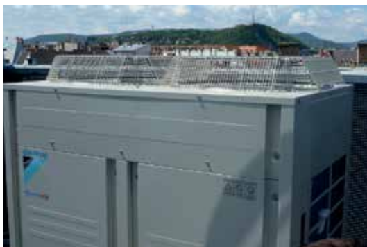
The compact and quiet outdoor units were installed on the store's roof, 30 m above the shop floor.
