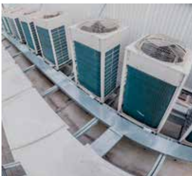
Eight VRV IV units serve 60 indoor units throughout the shopping mall.
