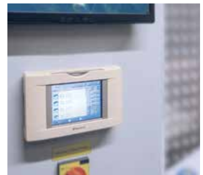
Daikin's simple controller ensures the integrated refrigeration and climate control system runs smoothly at all times.
