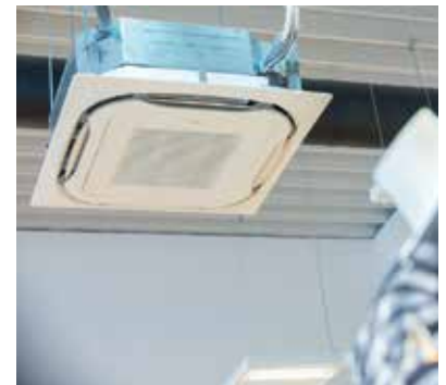
Self-cleaning ceiling units are used to heat all the stores.
