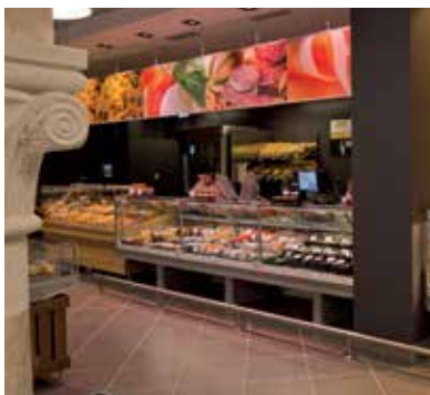
The system recovers waste heat from refrigeration to heat other parts of the store.
