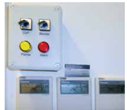
Daikin's user-friendly controls allow staff to control the shopping and office environments easily.
