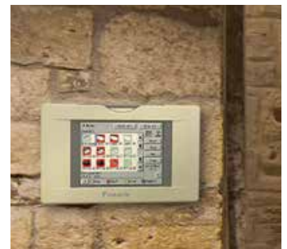
Daikin controls allow staff to control store comfort via an intuitive and user-friendly interface.
